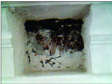
Fig 6. The corroding steel frame is revealed after opening up the stonework.
