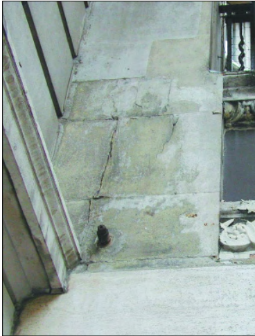
Fig 4. Cracking of stonework caused by corrosion of underlying structural steel frame.
